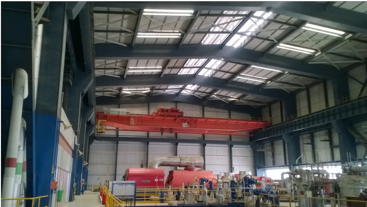
Figure 18. Overhead crane (Edipower – a2a Group).
